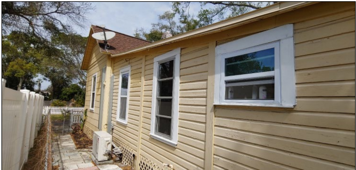
Figure 3: Photograph showing side elevation of addition to be removed. The ceilings do not appear to meet the minimum height required by Florida Building Code.
